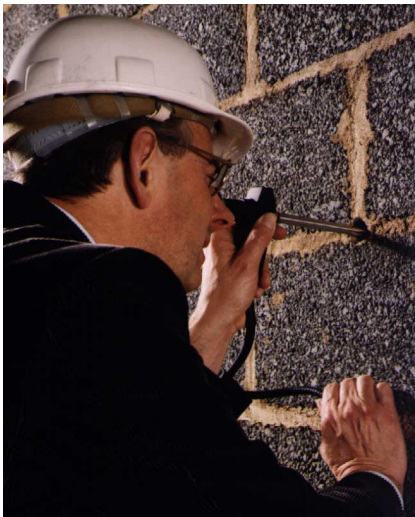
Using an optical probe to investigate hidden dampness in a cavity wall
