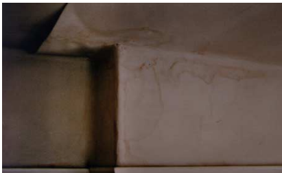
Staining to ceiling caused by rain penetration of chimney stack
