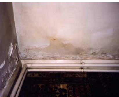
Typical rising damp stain on internal wall
