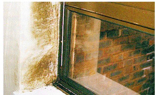
Typical example of mould caused by condensation
