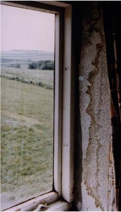
Rain penetration at a window jamb
