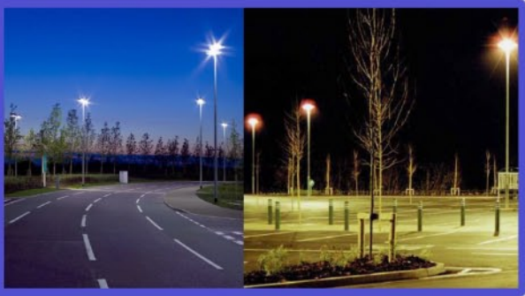
Example of roadway and carpark lighting
